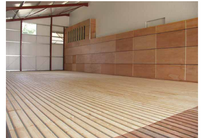
Vegetable store with ventilation and refrigeration fitted to a Lingward main air duct and floor.
