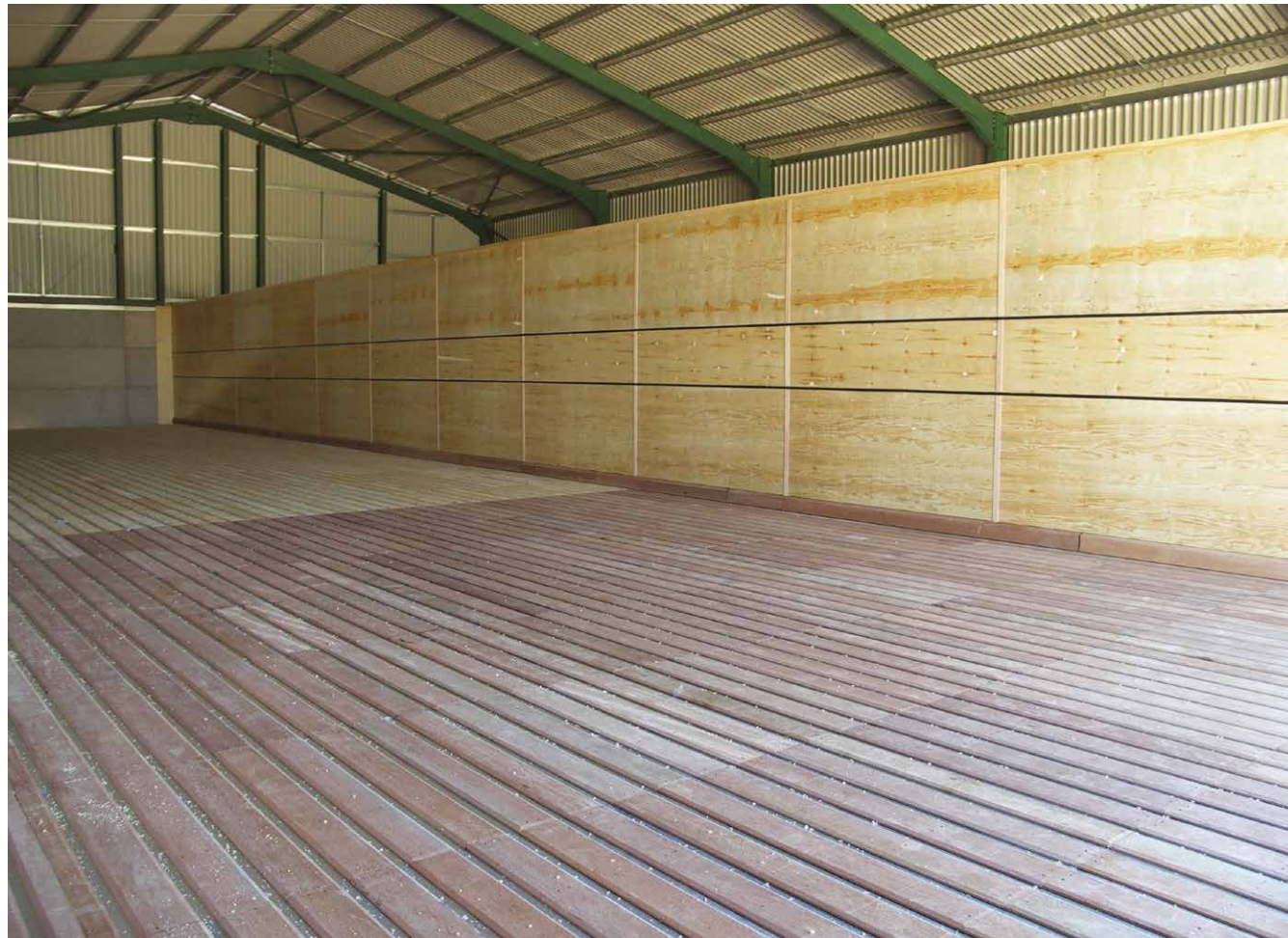
A composite hard and softwood Lingward floor fitted with a Lingward main air duct.
