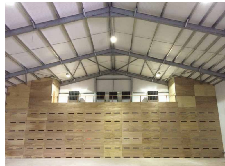
Suction wall for recirculation and ventilation in a box store.
