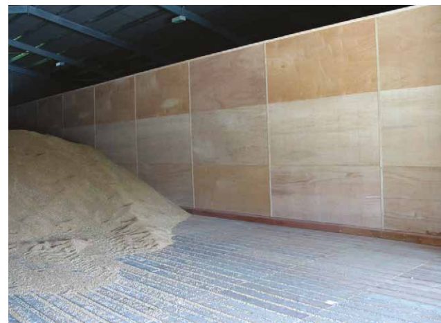
Drying floor with timber air duct
